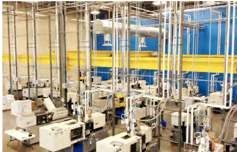
The lights-out injection molding machines that continually work to allow Eldon James to compete with offshore competitors
